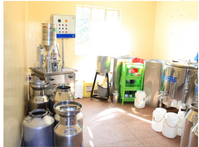
Figure 25: Vihiga Dairy Farmers Co-operative Cooling Plant (Day 2)
