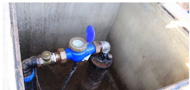
Figure 41: Mwibona Ward Water Project - Borehole
