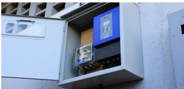
Figure 40: Mwibona Ward Water Project - Solar Energy Converter
