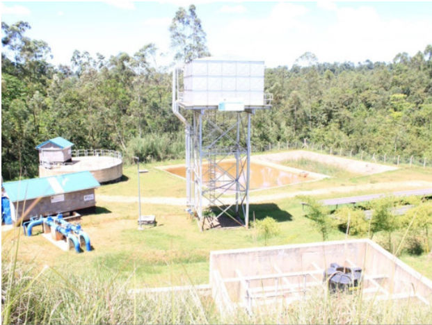
Figure 28: Lunyerere Water Scheme – existing water scheme and treatment facility (day 3)
