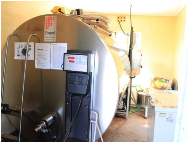
Figure 24: Vihiga Dairy Farmers Co-operative cooling plant - 10,000 litres milk cooling tank (day 2)
