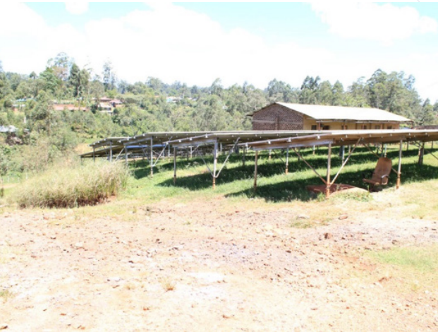
Figure 30: Lunyerere Water Scheme – solar panels (day 3)
