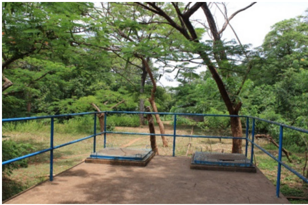
Figure 30: Water tank at Tavevo Water and Sewerage Company Taveta offices (day 3)
