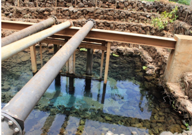
Figure 43: Njoro Kubwa Water Spring – existing water intake source
