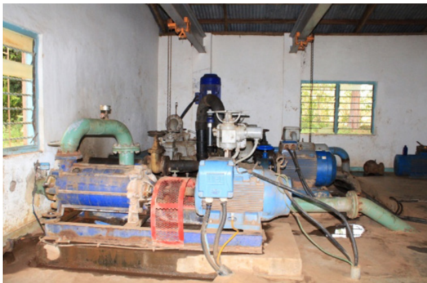
Figure 26: Water pumping equipment at the Taveta-Lumi Scheme (day 3)
