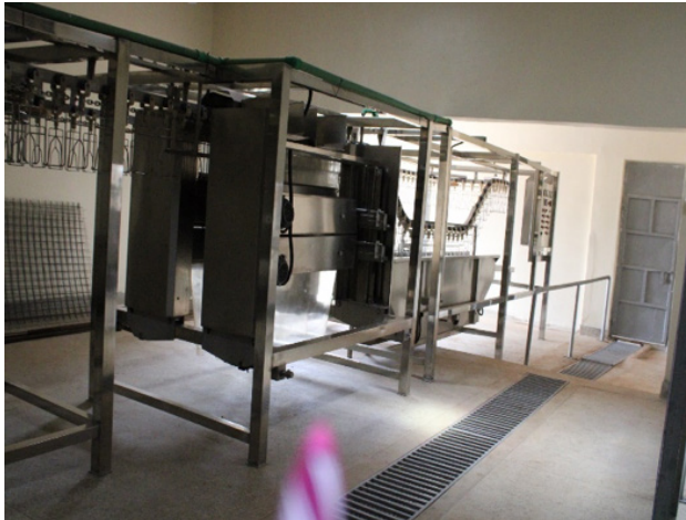
Figure 20: Site Visit to Poultry Slaughter House Kapsabet (day 2) – installed equipment.
