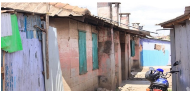
Figure 47: County government houses in Bahati Estate that have been earmarked for redevelopment
