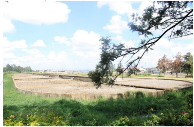
Figure 43: Kariobangi Sewerage Treatment Plant - Sludge drying pits
