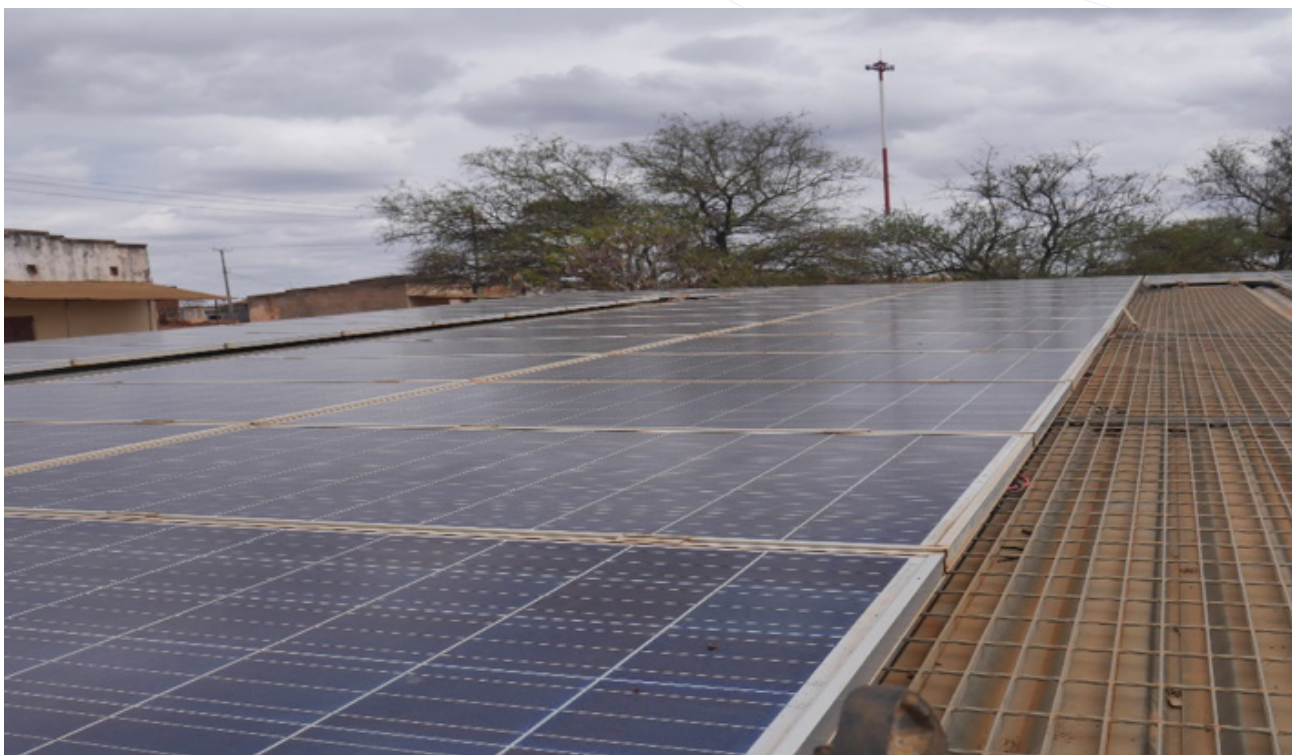
Figure 39: Solar panels at the Kitonyoni solar plant
