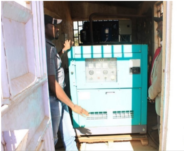
Figure 44: Electricity supply house at the Muhotetu milk cooling facility
