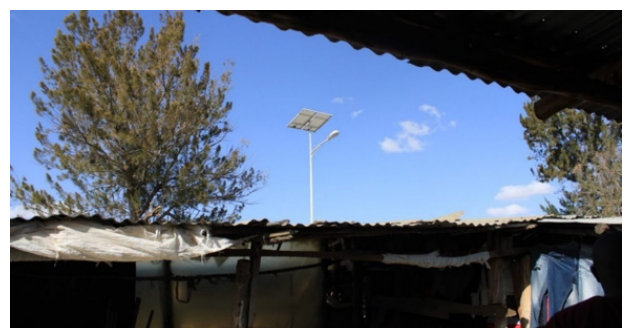
Figure 46: Non-functional solar power lighting at the Mutumba Market
