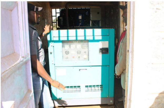
Figure 27: Power House at Muhotetu Dairy Farmers Co-operative Society cooling plant (Day 3)
