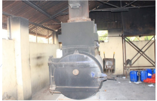
Figure 23: Embu Level 5 Hospital - incinerator for burning medical waste (day 3)
