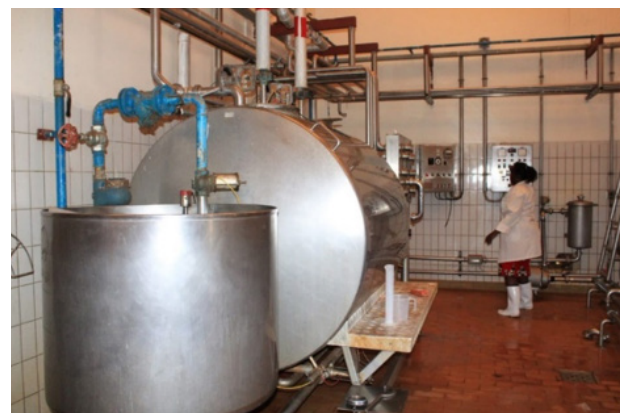
Figure 47: Runyenjes Milk Cooling Plant - cooling tanks
