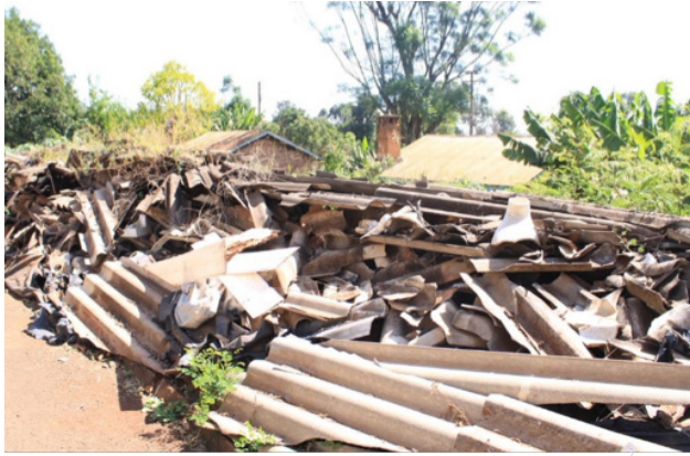
Figure 22: Embu Level 5 Hospital - asbestos waste from replaced roofing (day 3)
